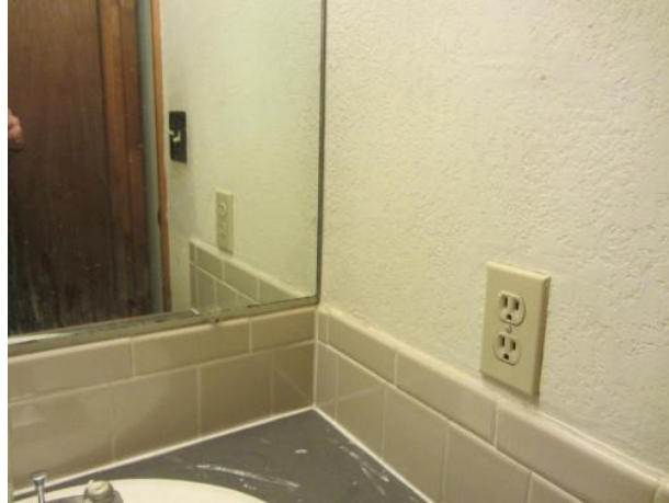
Figure 3: Non-GFCI outlet within 6’ of sink in bathroom.
