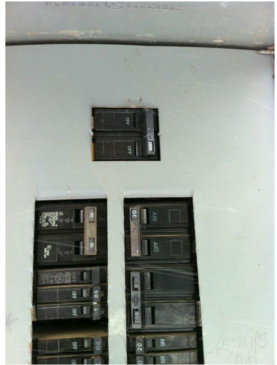
Figure 6: Readily accessible panel.
