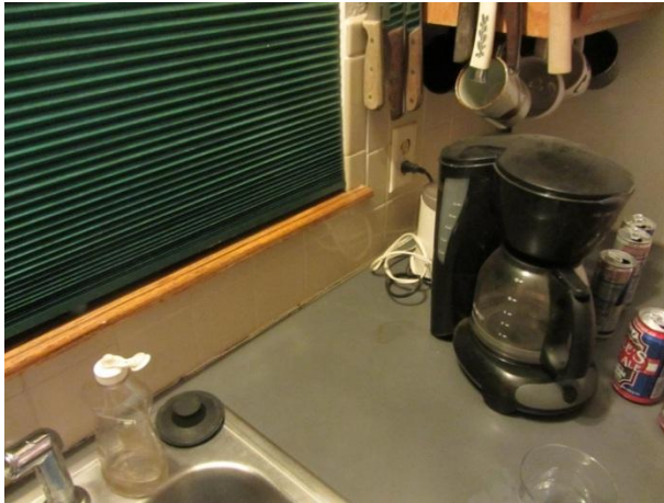
Figure 2: Non-GFCI outlet within 6’ of sink, in kitchen
