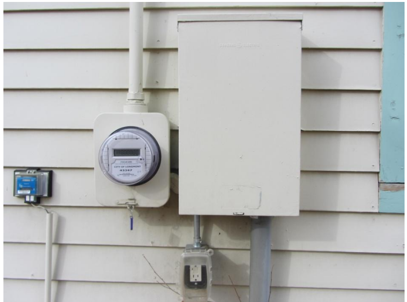
Figure 1: Panel and Meter
